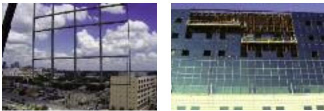
Baylor All Saints Medical Center, Fort Worth, TX Architect: Gideon Toal, Inc., Fort Worth, TX Glazing Contractor: DGB Glass, Fort Worth, TX Construction photos courtesy of DGB Glass
